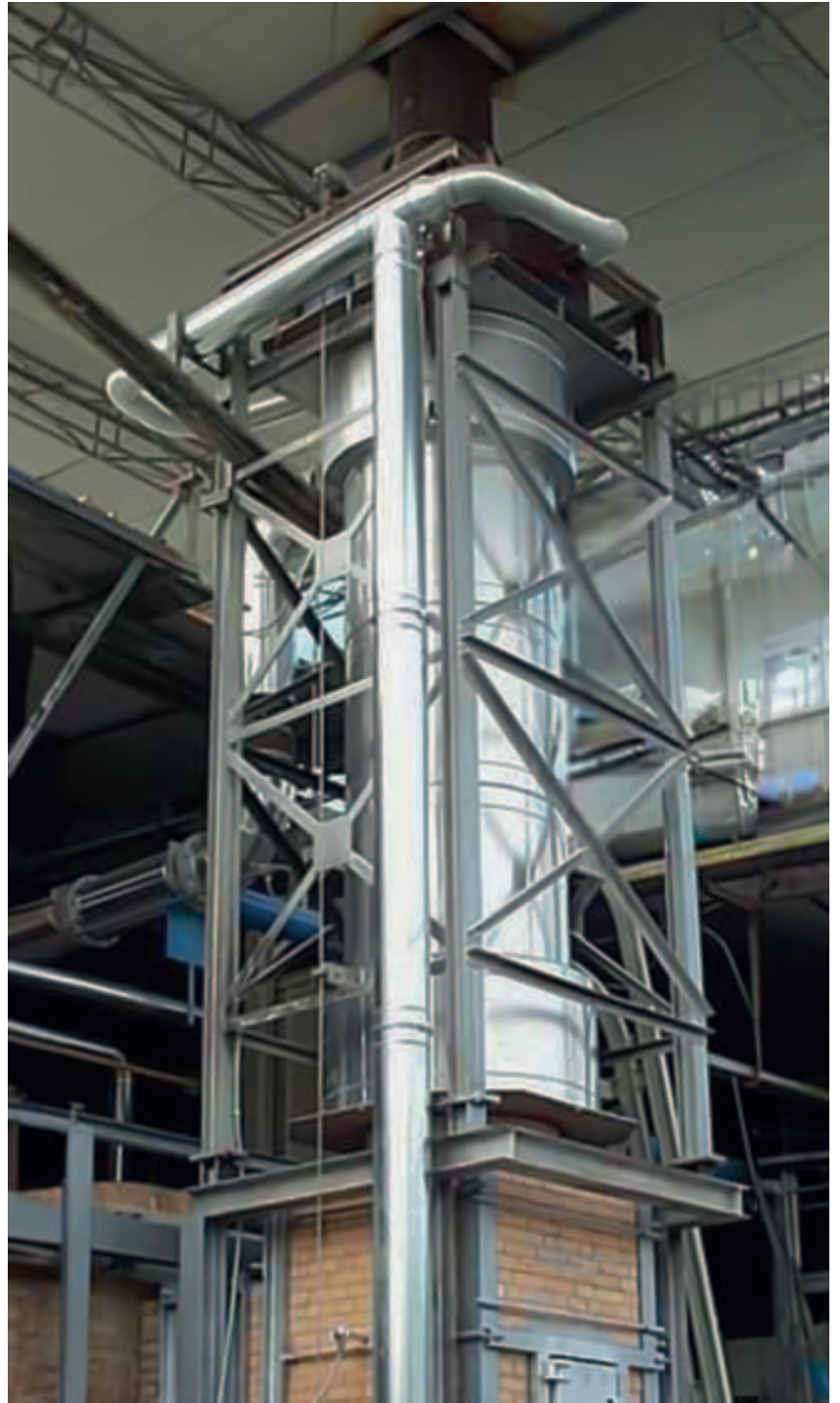
Typical configuration with double stage recuperator
